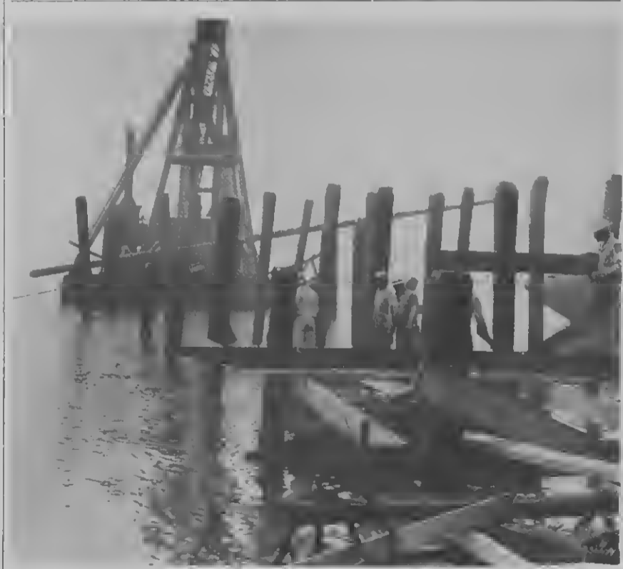
MECHANICAL Department forces went to work last month driving piling for the crude pier which will replace the old Lake Tanker Docks. Each pile is 75 feet long and tapers from seven inches in diameter at the tip to 18 inches at the butt. They will support the 755-foot-long pier which will handle two 26,000-deadweight-ton tankers. Completion date is expected about Sept. 15.
